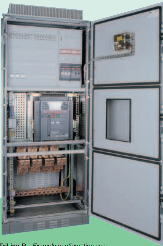
TriLine-R – Example configuration as a power distribution board
